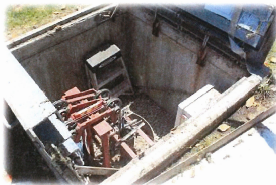
Ground Level Monitoring Equipment at Ayala Park
